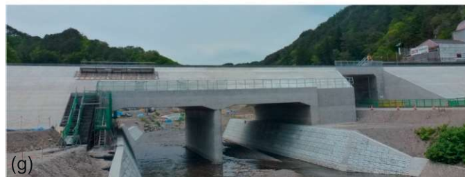
Figure 23.29 cont'd (c) embankment seen from the inland side (May 20, 2014); (d) GRS integral bridge; (e) immediately after earthquake (March 30, 2011) seen from the sea side; (f) GRS integral bridge and RC box culvert during construction (June 19, 2013); and (g) completed (May 20, 2014) at Shimanokoshi Station, Sanriku Railway.
