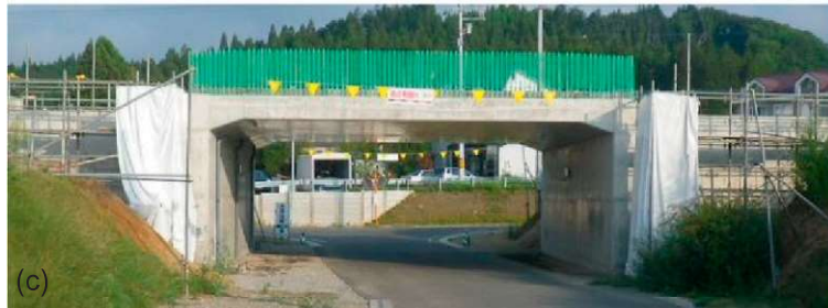
Figure 23.19 GRS integral bridge at Kikonai, Hokkaido Shinkansen (at site I in Fig. 23.7(b): (a) details, (b) during construction (October 14, 2011), and (c) completed (July 31, 2012).
