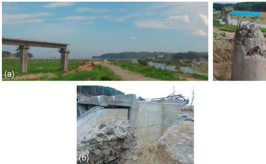
Figure 23.25 (a) Tsuyano-kawa bridge at JR East Kesenu-numa Line that lost multiple simple-supported girders as a result of tsunami forces; and (b) a view of the back of the right bank abutment of Yonedagawa bridge at Noda, Iwate Prefecture, North Rias Line, Sanriku Railway.
