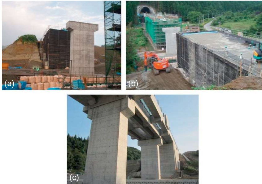
Figure 23.16 GRS abutment at Mantaro for the Hokkaido Shinkansen (A21 in Fig. 23.7 (b)—views under construction: (a) from the front side, (b) from the backside, and (c) completed. (Source: From Yonezawa et al. (2013, 2014)).
