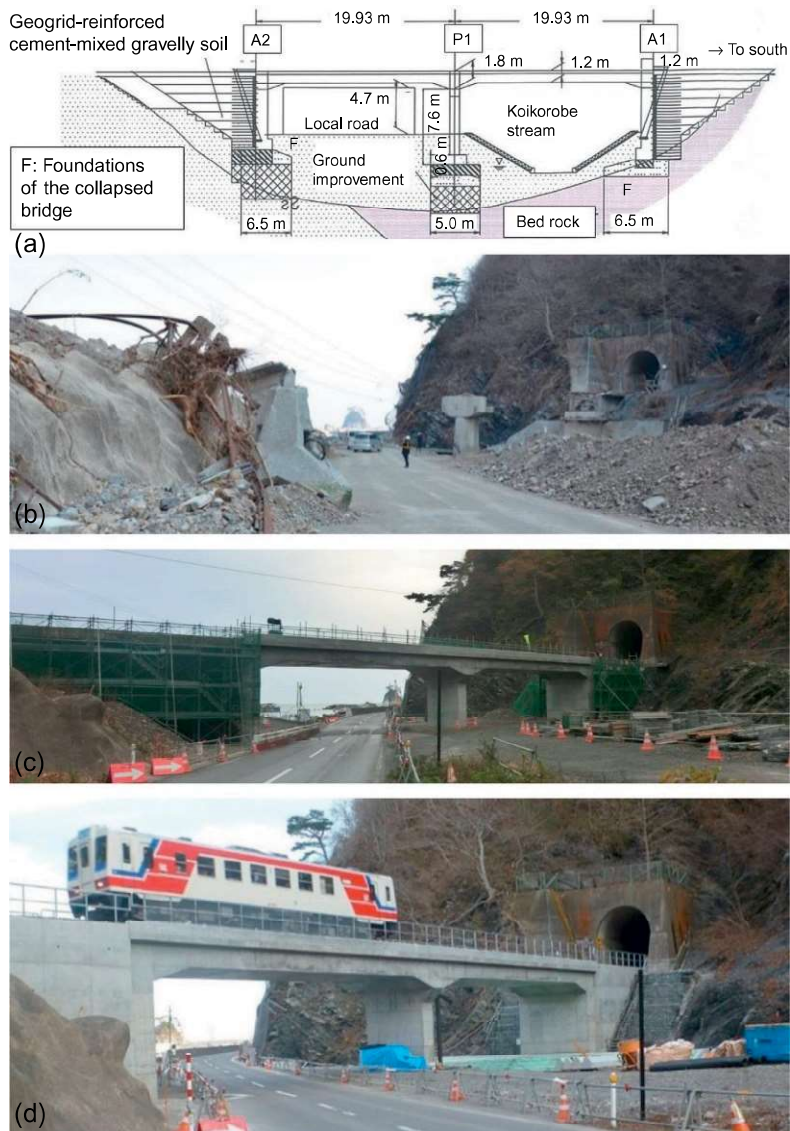
Figure 23.27 (a) Plan of GRS integral bridge seen from the inland side; (b) immediately after collapse (March 30, 2011); (c) under construction (November 3, 2013); and (d) completed (April 6, 2014) at Koikorobe, Sanriku Railway.
